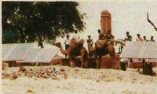
XI. 2 Solar Powered Pumping System installed by CEL at Churu, Rajasthan under the National Drinking water Mission.
