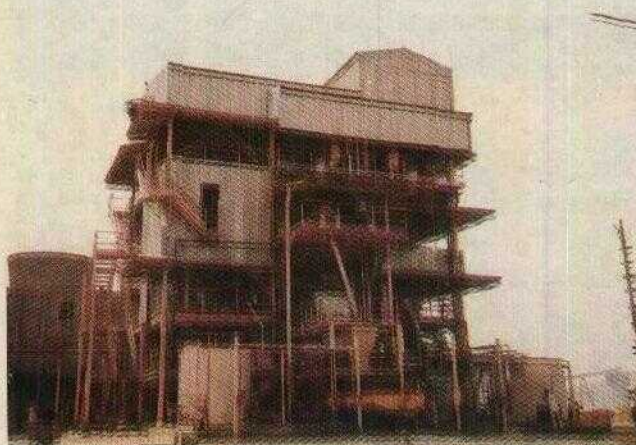
IV. 3 Cryolite Recovery Pilot Plant.
