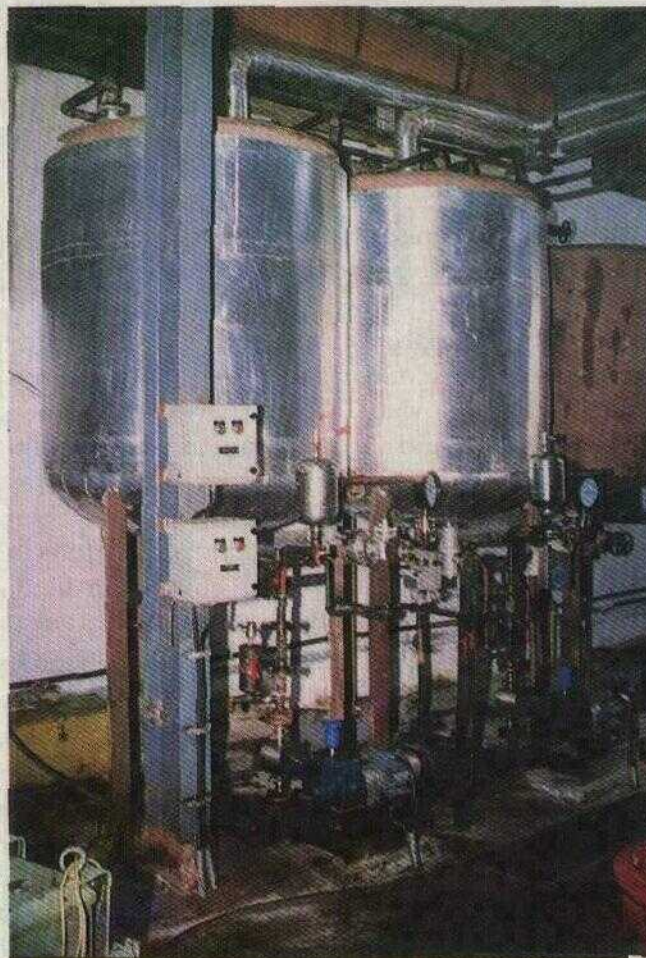
V.C.1 Distillation Tank in M/s Balmer Lawrie Pilot Plant
