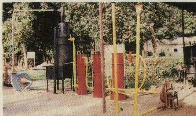
III.B.4 220 KW Rice Husk Gasifier System
