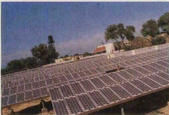
VII.B.1 View of SPV Array 100 KW Power Plant at Kalyanpur, Distt. Aligarh, U.P. for NEDA
