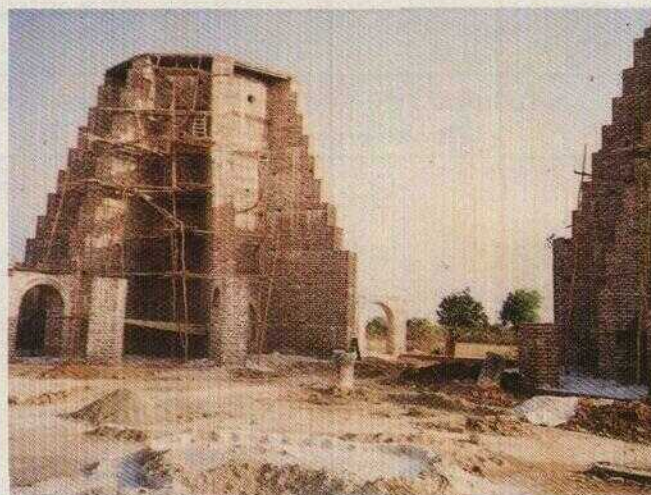
II. 3. Erection of Control System and Lime Kiln at Aditya Lime Industries, Ramtek
