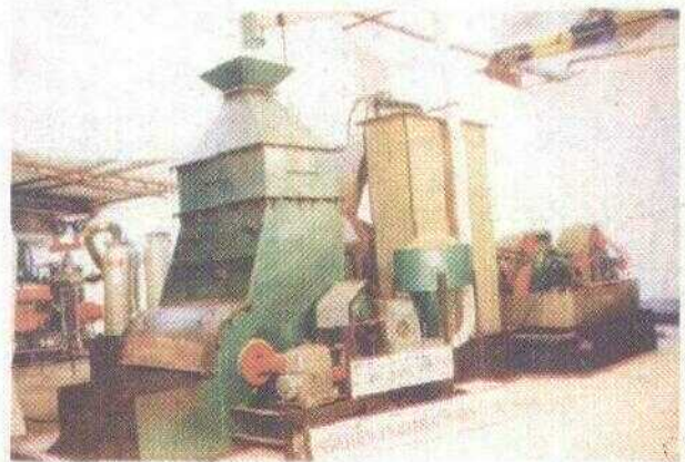
III.A.2 100 KW Rice Husk Gasifier
