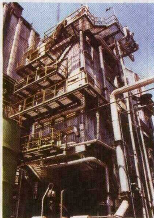
III.A.3 Waste Heat Recovery Steam Generator
