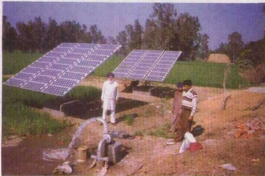
VIII.B.1 SPV Water Pumping System by CEL in a village in Punjab
