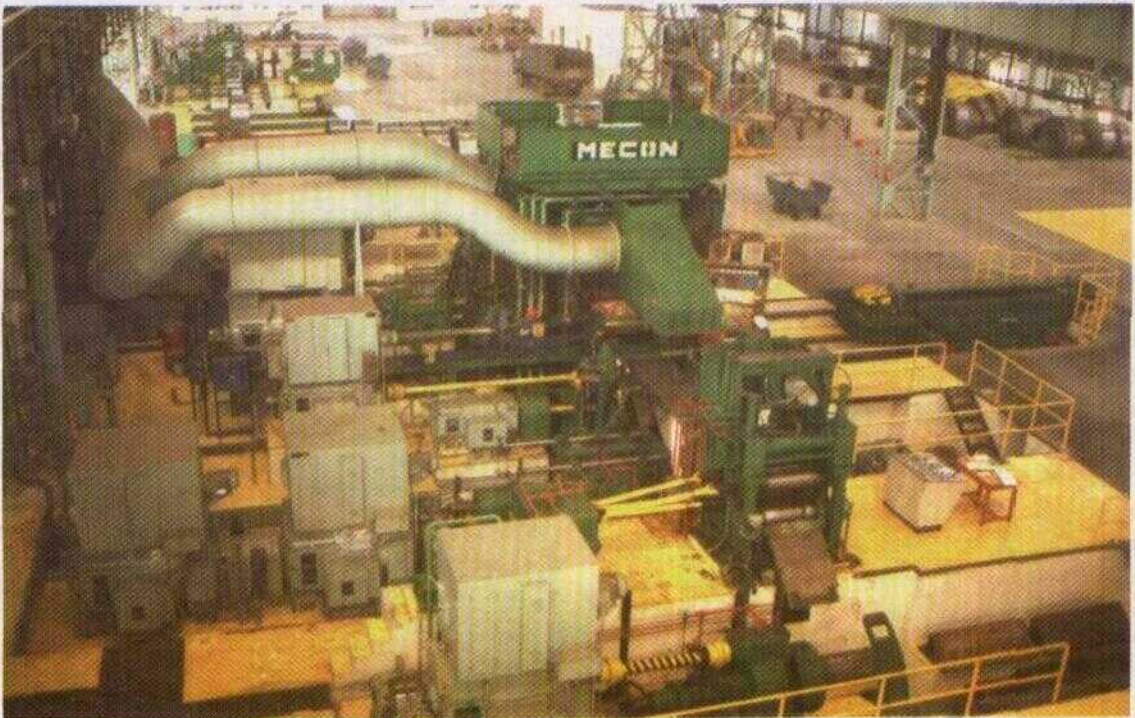
III.A.1 Overall side view of 6 High Rolling Mill
