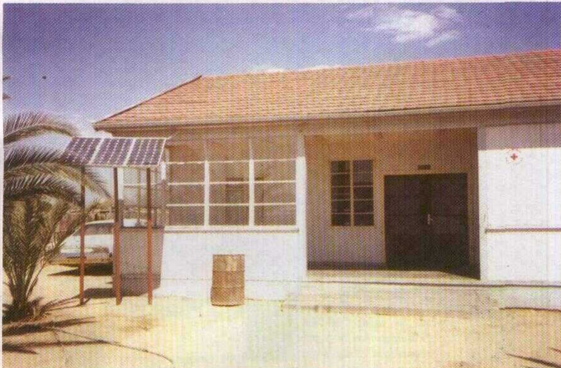
VIII.B.2 SPV Powered Lighting of Medical Centre by CEL in Village Spitzskoppe in Namibia
