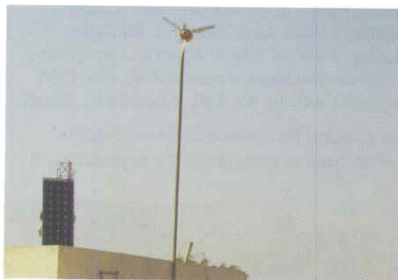
Prototype Small PV-Wind hybrid power plant for rural application
