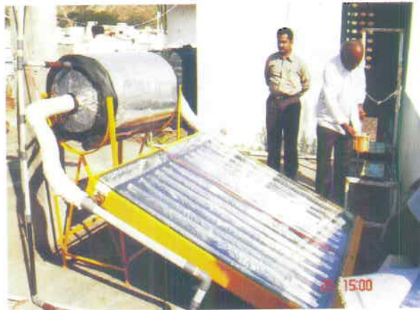
Solar Water Heater with fused tube lights
