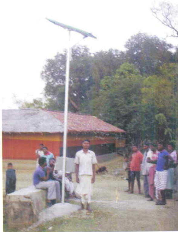
SPV Street Lighting System in a Remote village of Jharkhand
