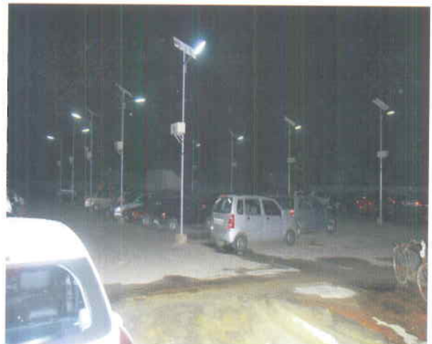
Solar Street Lights in Parking area of Patel Chowk Station of Delhi Metro Rail Corporation Ltd
