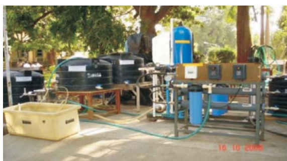
Fig 81: RO hybrid plant for the treatment of feed water and reject water containing excess Fluoride
