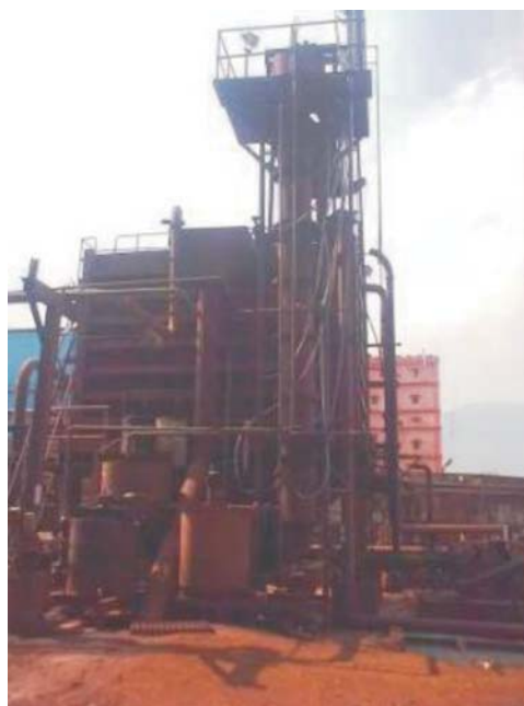
Fig 85: Pilot plant – 0.6 m diameter flotation column
