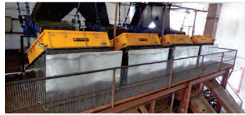
50 - 13 mm modules at GMDC Lignite Beneficiation Plant
