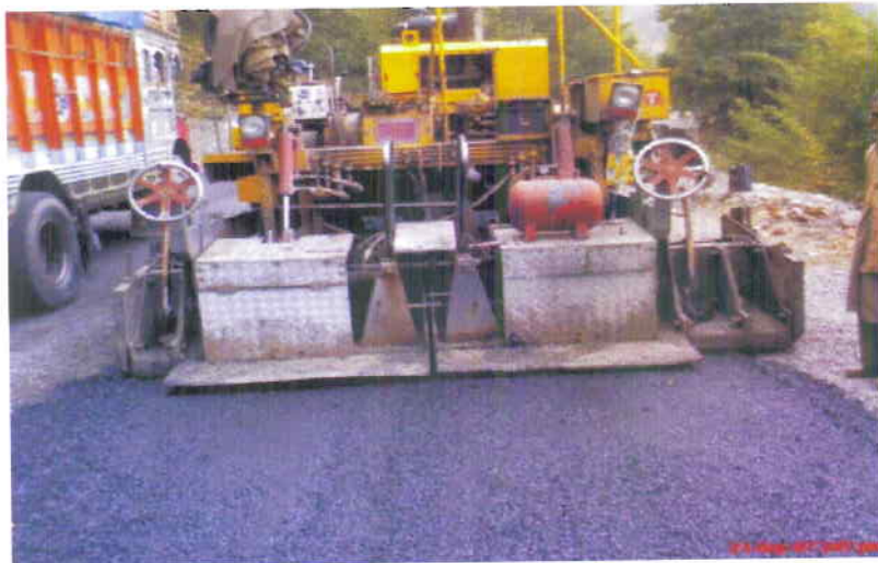
View of construction with environment friendly emulsion based cold mix technology on Jammu-Srinagar road (NH-1A) in snow bound area
