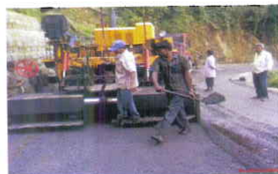
View of construction with environment friendly emulsion based cold mix technology in Aizwal city in Mizoram in high rainfall areas
