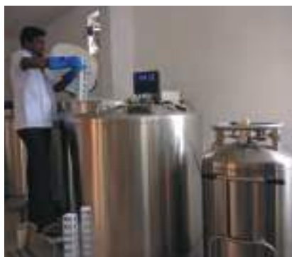
▲ Liquid nitrogen storage facility
