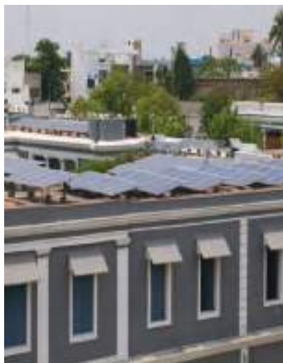
Smart grid-tied solar power plants on the rooftop of the Ashram buildings using net electricity metering
