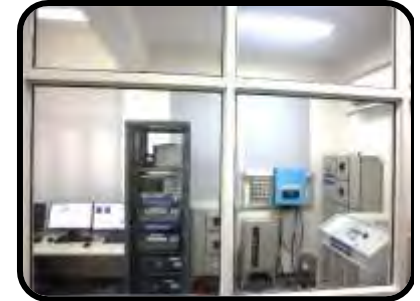
Grid Tied Inverter Test Facility
